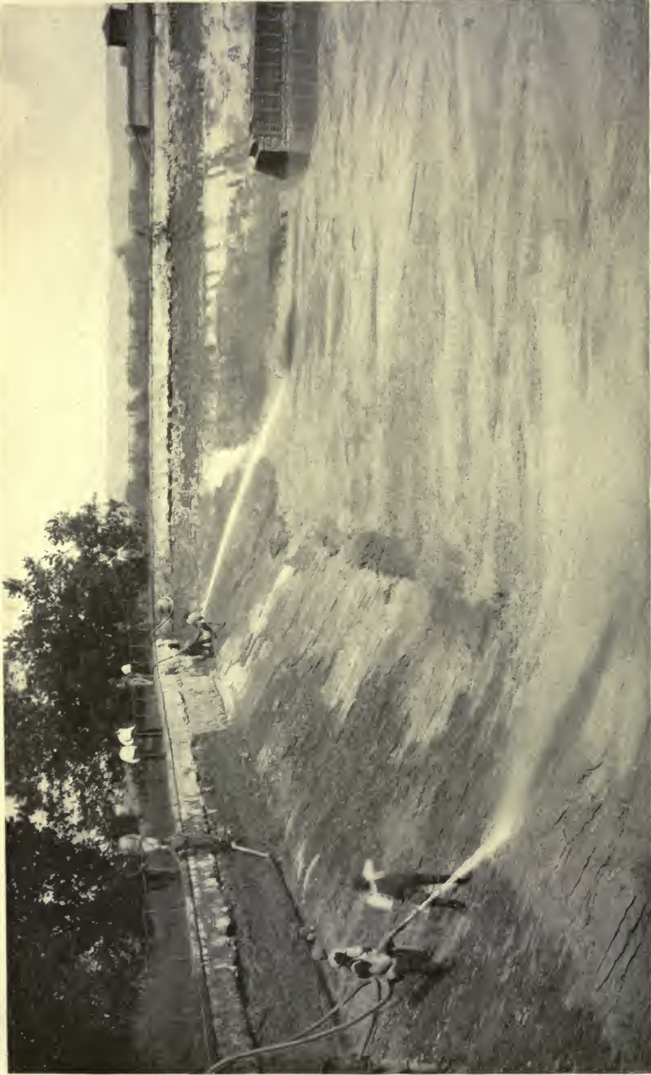
REMOVING MUD FROM THE SECONDARY SETTLING BASINS AT THE STORAGE RESERVOIRS OF THE LEAVENWORTH WATER COMPANY
