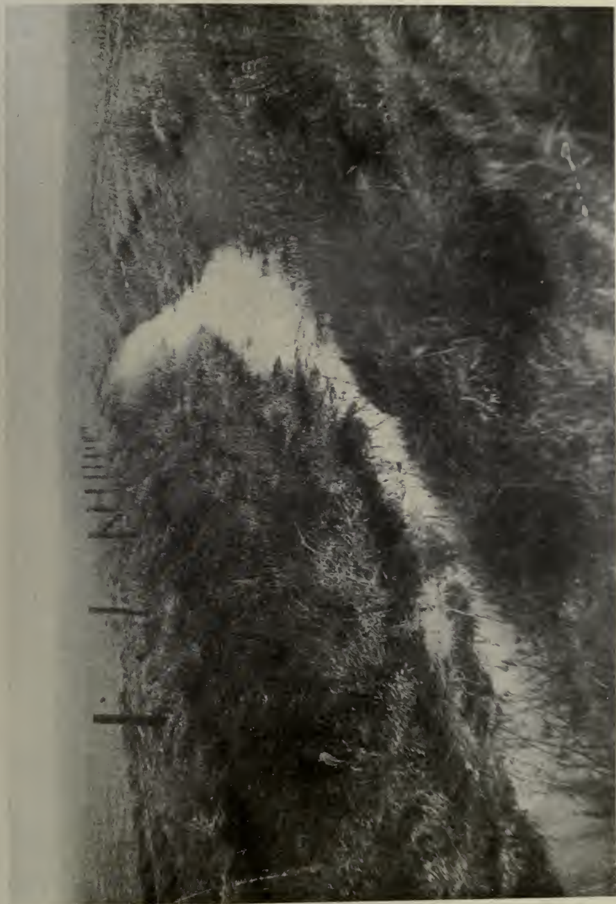
A POORLY CONSTRUCTED DRAINAGE DITCH—SIDES CAVED AND ERODED
