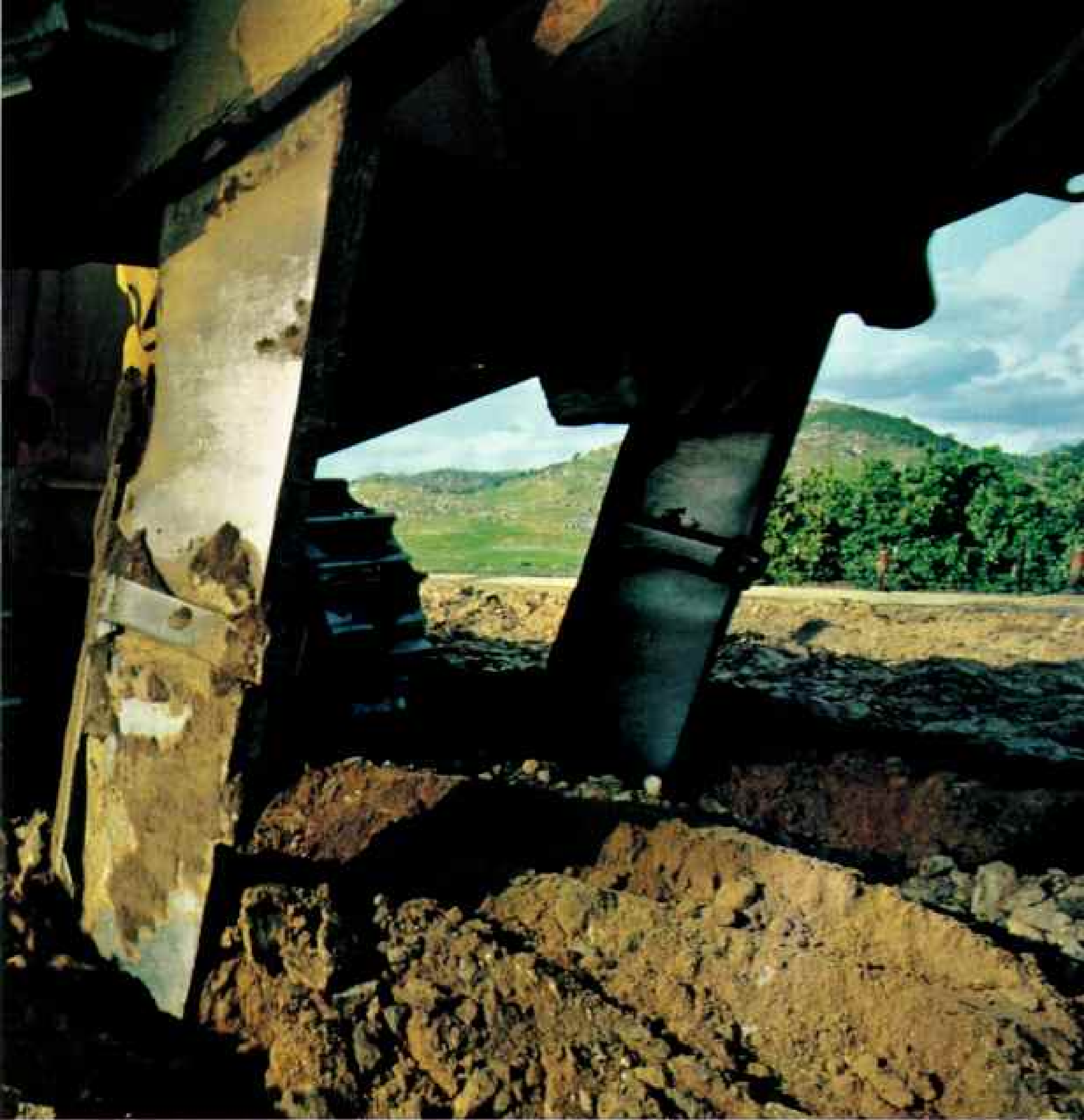
RIPTING THROUGH CALIFORNIA HARDPAN, SOIL ENGINEERS MAKE WAY FOR A CITRUS GROVE.
