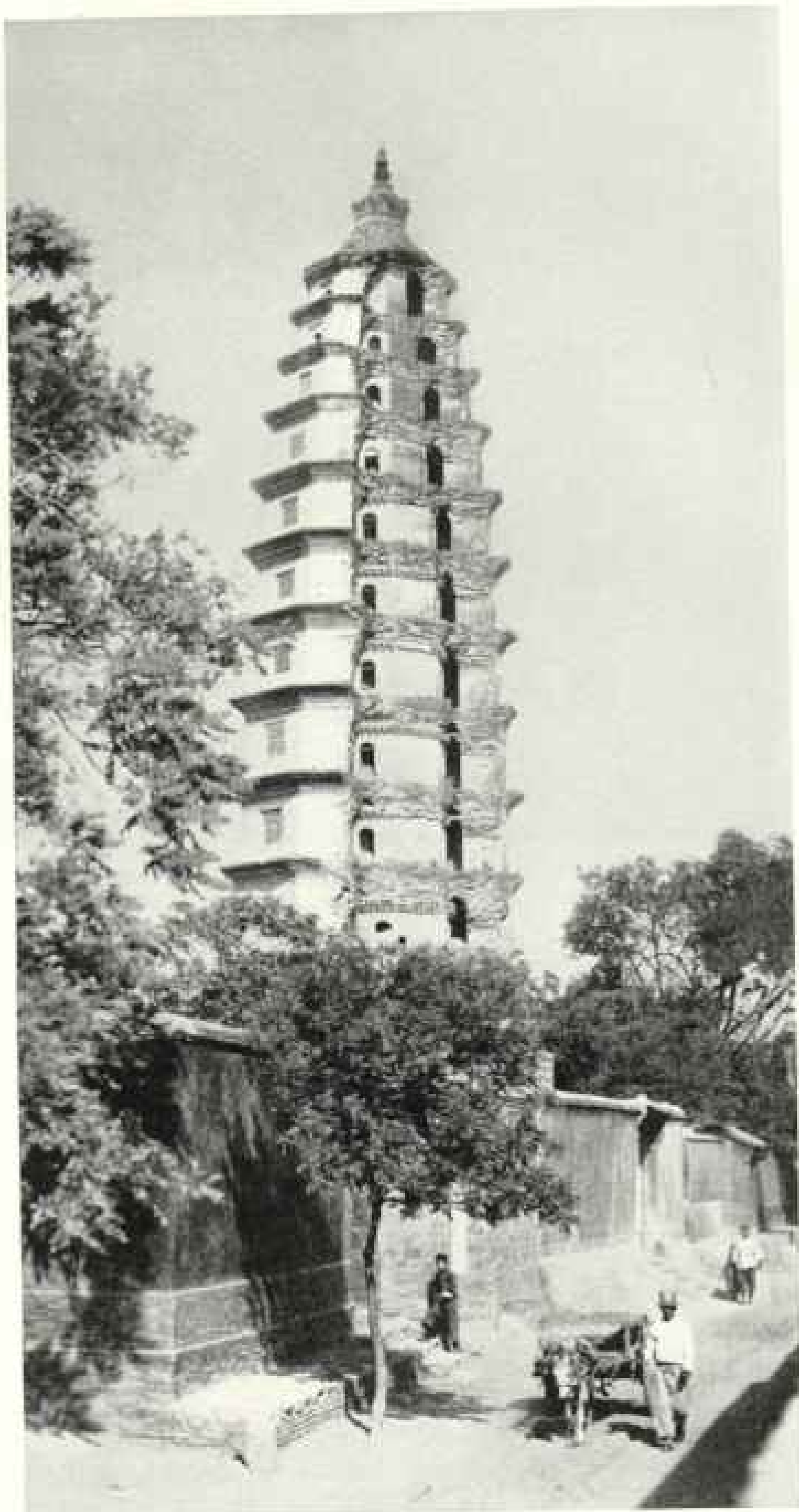
ONE SIDE OF THIS PAGODA FELL AWAY, REVEALING AN OLDER STRUCTURE INSIDE
