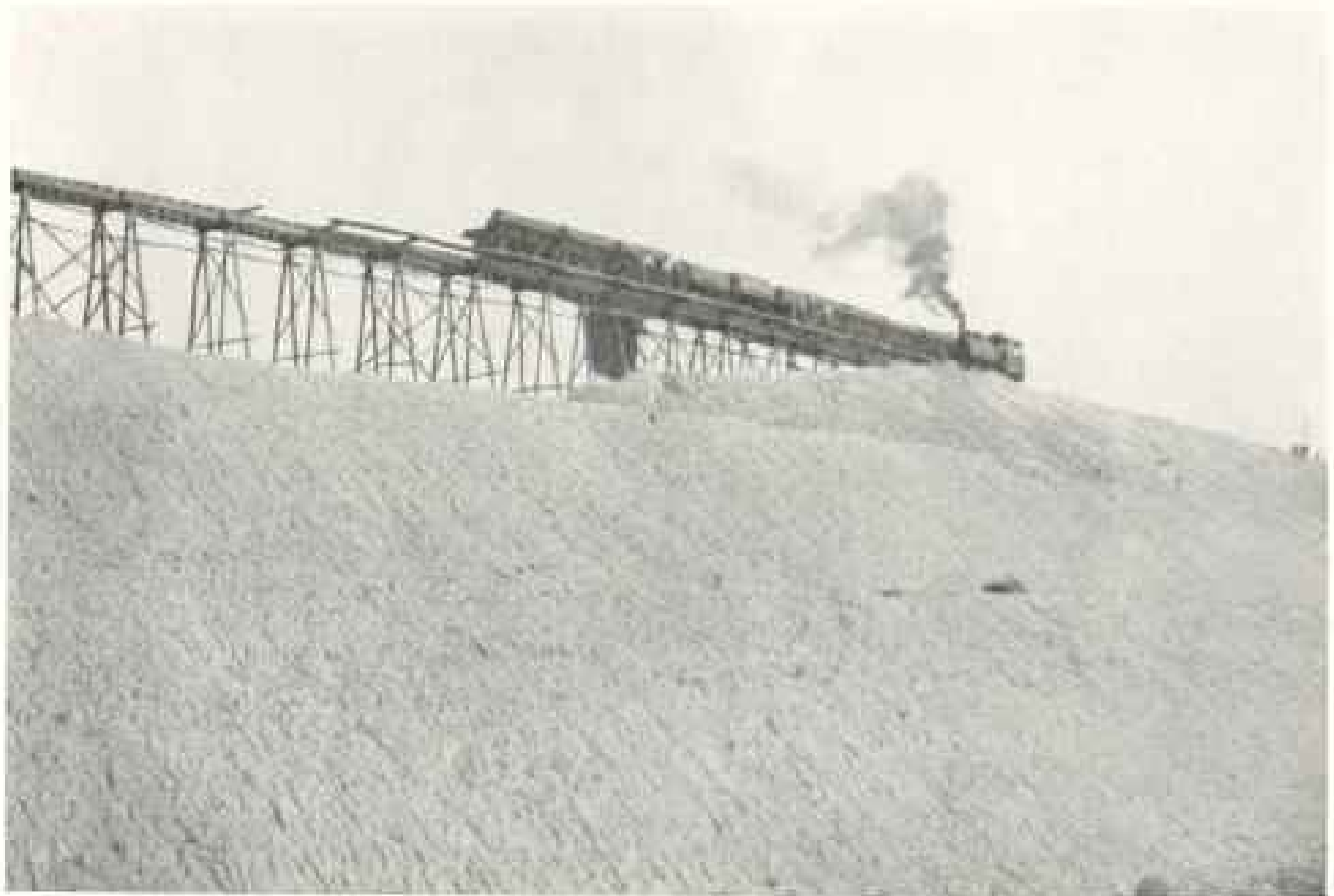
BUILDING THE EMBANKMENT APPROACH TO THE BURLINGTON'S BRIDGE ACROSS THE OHIO RIVER AT PADUCAH, KENTUCKY
