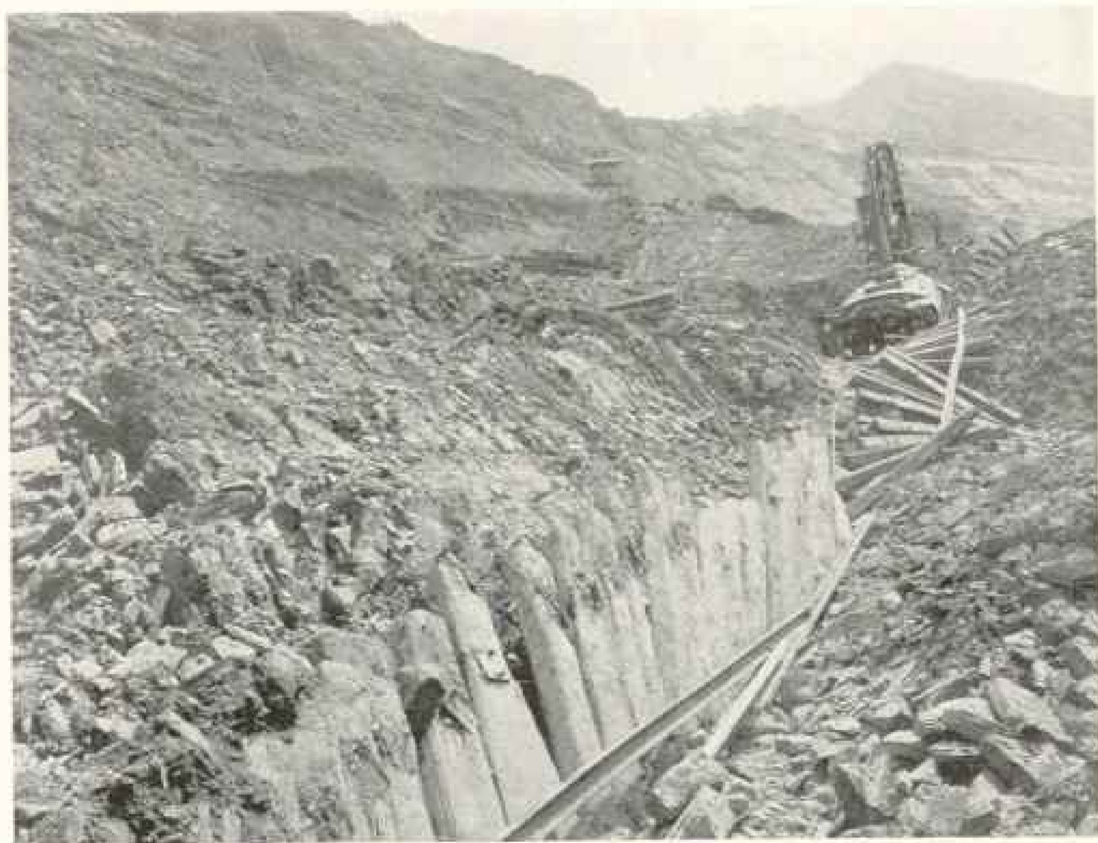
A STEAM SHOVEL HALF BURIED BY A SLIDE
