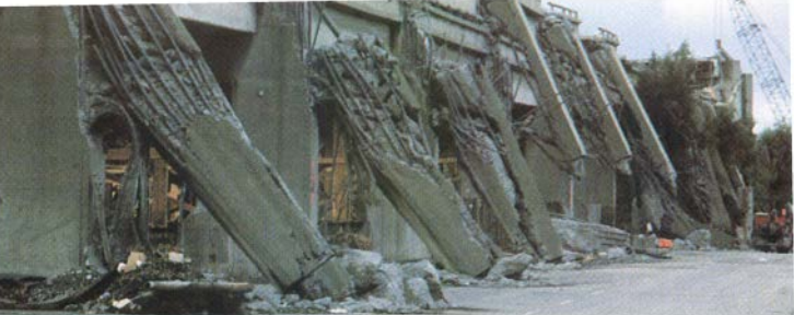
Destruction caused by the California earthquake of October, 1989
