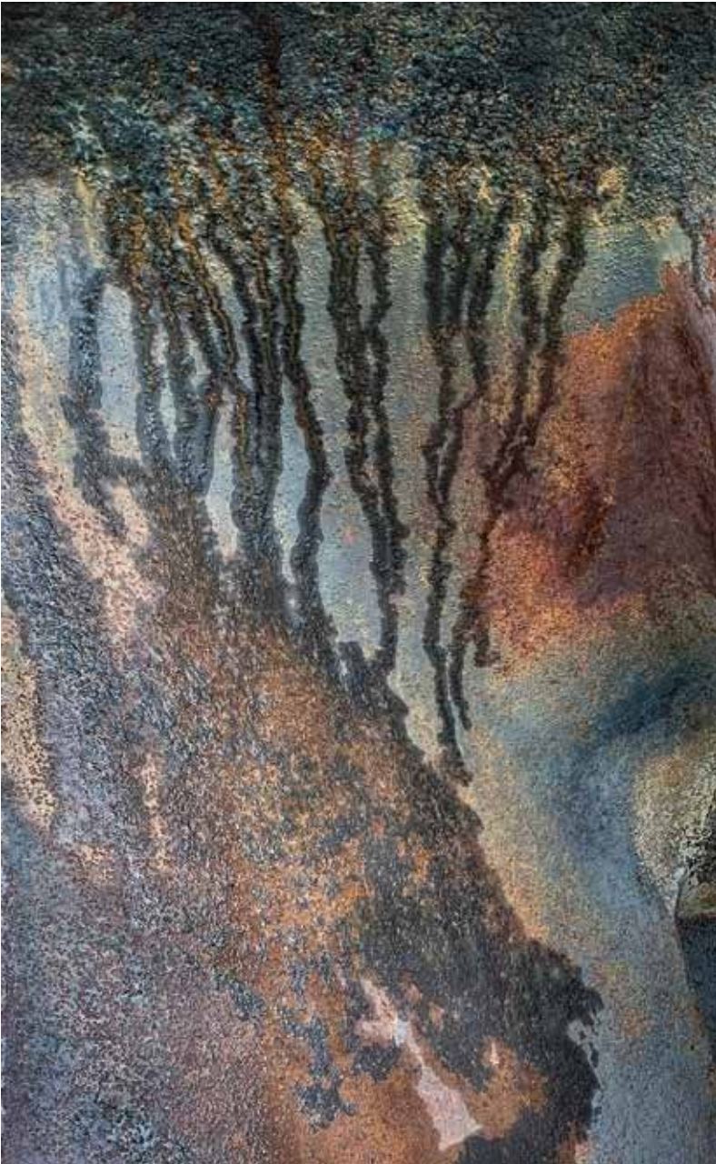
Figure 23.2 Close detail of corrosion and rain water.
