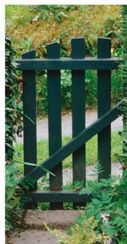
GAPS UNDER GATE
