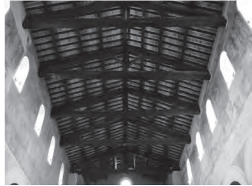
319. San Giovanni a Porta Latina, Rome. Exposed ceiling with a view of the gable roof trusses and underside of the roof tiles
