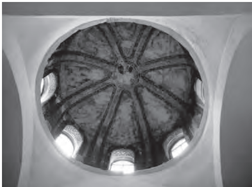
410. St Theodore, Constantinople. Narthex dome and drum with original Christian figures faintly visible
