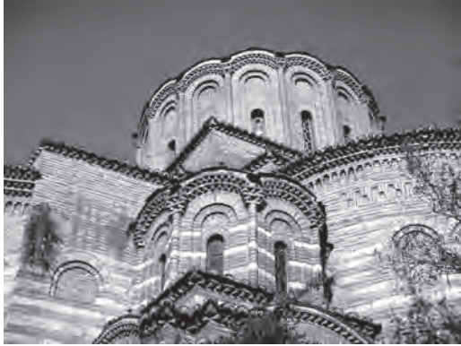
518. Prophet Elijah, Thessaloniki. View from the northeast corner showing three sides of the prothesis drum and dome (centre front) and tall arched drum of the central naos dome (centre back)
