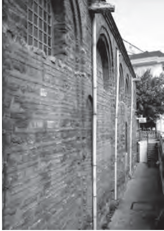
383. Theotokos Panachrantos, Constantinople. Side wall of the parekklesion showing a stair down from present day ground level
