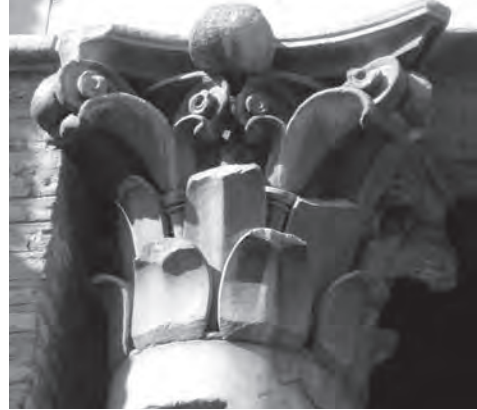
264. SS Giovanni e Paolo, Rome. Unusual simplified Corinthian capital in end column of portico
