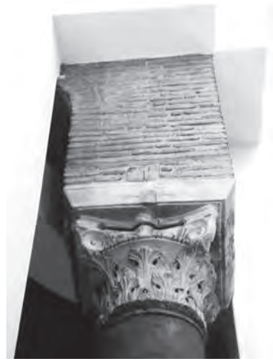
522. Prophet Elijah, Thessaloniki. Reused classical column and lower portion of original arch left exposed
