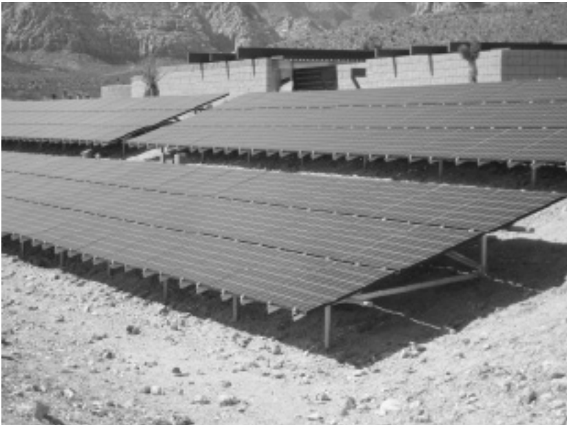
Figure 10-4. Solar Electric Array at Red Rock Canyon Visitor Center
