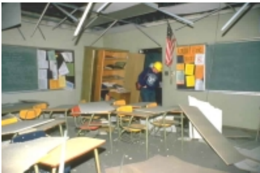
Federal funds may be used to repair or replace disaster-damaged public facilities, such as schools.
