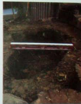
A carpenter's spirit level shows if both sides of the excavation are at the same level.
