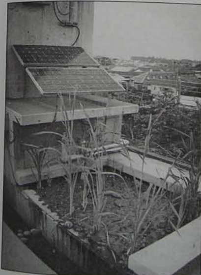
Photo 13.6: Solar powered grey water system.
