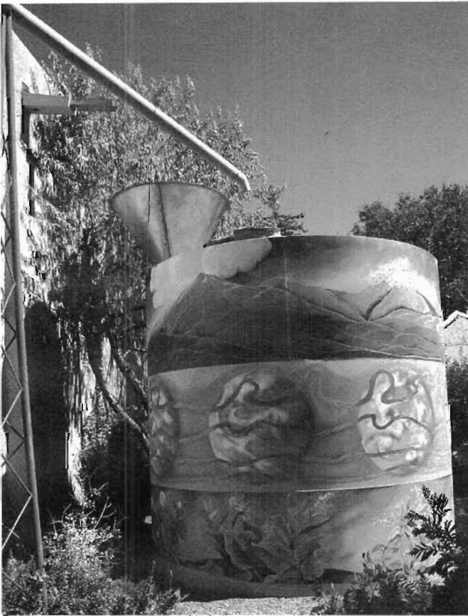
Fig. 3.31. A 10,000-gallon (37,850 liter) steel tank/mural and dry system downspout collecting roof runoff for irrigation, Children's Museum, Santa Fe, New Mexico. A dry system downspout drains all water out of the pipe, leaving it dry between rains. It does not collect sludge nor is it prone to freezing damage.
