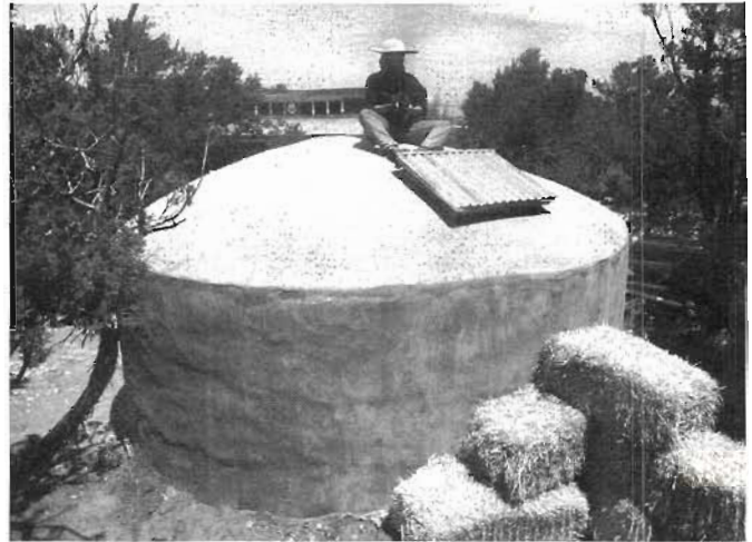
Fig. 3.36. A 6,000-gallon (22,700-liter) ferrocement tank storing roof runoff for domestic use and irrigation, Meuli residence, Tijeras, New Mexico. The square piece of corrugated metal atop the tank is the lid to the access hole.
