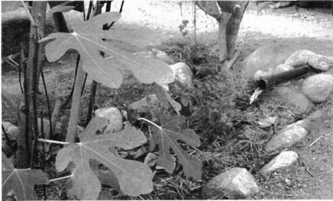
Fig. 4.27. Each greywater drain outlet is placed in a mulched and vegetated infiltration basin that also harvests rainwater and runoff. The pipe discharges, or outlets 3 inches (7.6 cm) above the mulch so roots do not grow into, and clog the pipe. The greywater immediately infiltrates beneath the surface of the mulch. Greywater is dispersed to multiple basins to reduce flow to any single basin, thus infiltration is further enhanced. The basins are also sized to contain and infiltrate several times the peak surge of greywater that will be discharged in a short period of time. For more info and additional variations see the Greywater chapter of volume 2.
