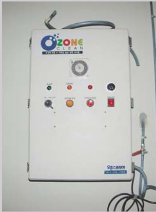
Figure 10. Ozone generator attached to the outside wall of the inoculation room
