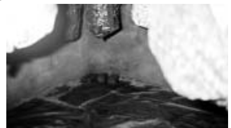
Figure 11. Mushroom house floor without sand. Water flooded onto the floor directly
