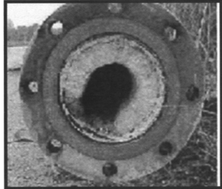
(f) Pipe fouled with struvite
