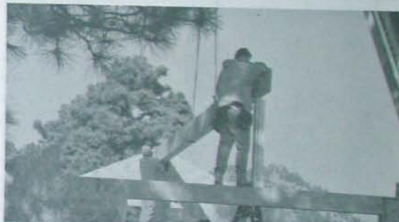
Fig. 1.9: Seeing the roof beams lifted into place seems magical. Now I remember why I love building! Credit: David Johnston.
