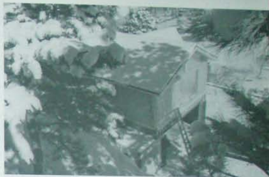
Fig. 1.11: After we had waterproofed the roof, it snowed for a month. Credit: David Johnston.
