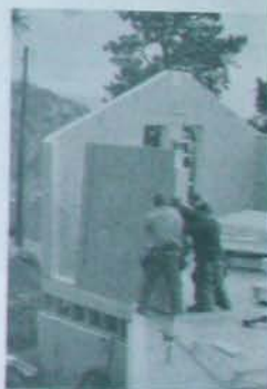
Fig. 1.7: This temporary panel madness will transform into roof and walls. Credit: David Johnston.
