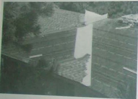
Fig. 1.10: The roofing membrane (typically made of felt paper), keeps water out of the roof, the white flashing keeps moisture out of the roof valley, and 50-year composition shingles protect the roofing membrane from sunlight degradation.
