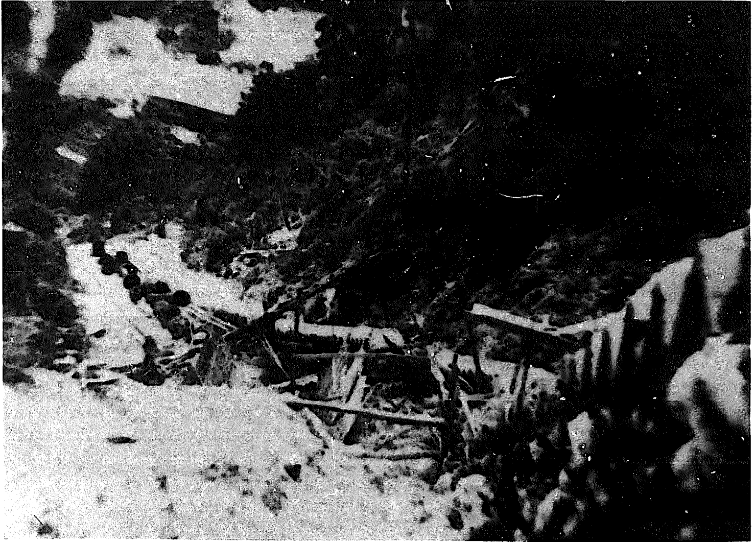
Route of penstock pipes for the Hanga-Hanga plant with work in progress. The conditions, limestone rocks and a relatively steep inclination, make a heavy construction necessary. Soil investigation was by test pits.
