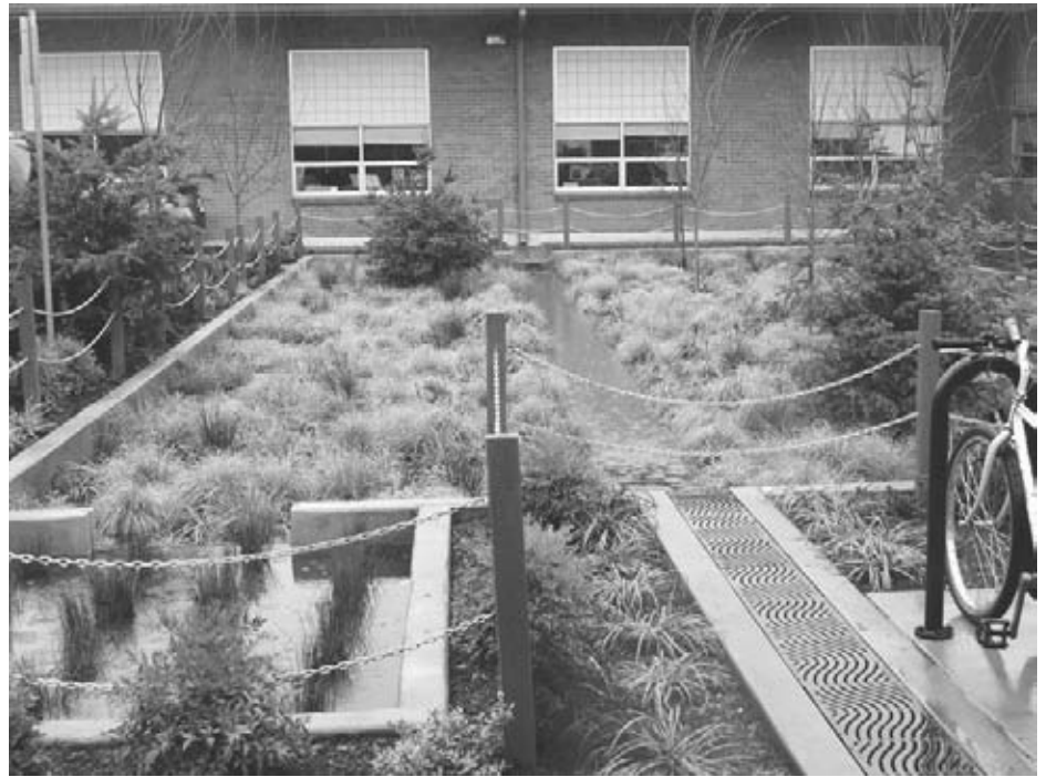
Figure 4.64 The Mount Tabor Middle School Rain Garden took a small school parking lot and converted it into a garden where children can learn about sustainable water practices. Image courtesy City of Portland.
