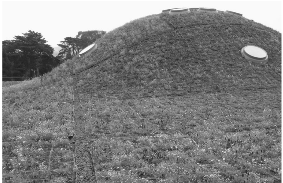
Figure 4.51 The green roof consists of a series of undulating “hills” that include skylights. Image courtesy California Academy of Sciences.
