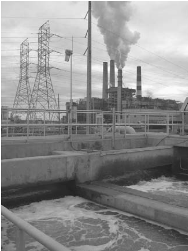
Figure 4.87 The Tampa Bay Seawater Desalination Plant cost $158 million to construct. Image courtesy Treehuggers.org.
