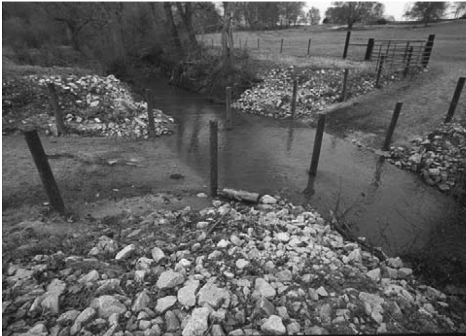
Figure 2.23 Allowing livestock in a stream can have a negative impact on water quality and riparian habitation. The use of a concrete water crossing allows livestock to cross the creek with minimal impact. Image courtesy NRCS.
