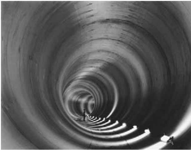
Figure 3.44 The Singapore Deep Tunnel Sewerage System utilizes cutting-edge technology to address the city's sanitary sewer problems. This image shows one of the two large tunnels that are each more than 80 kilometers (30 miles) long and up to 6.5 meters (7 yards) in size. Image courtesy Public Utilities Board of Singapore.
