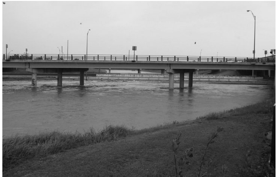
Figure 3.83 Brays Bayou uses multiple techniques to address flood risks, including channel modifications, bridge modifications, and the construction of regional stormwater detention basins. More than 70 individual projects have been implemented along the bayou. Image courtesy U.S. Army Corps of Engineers.
