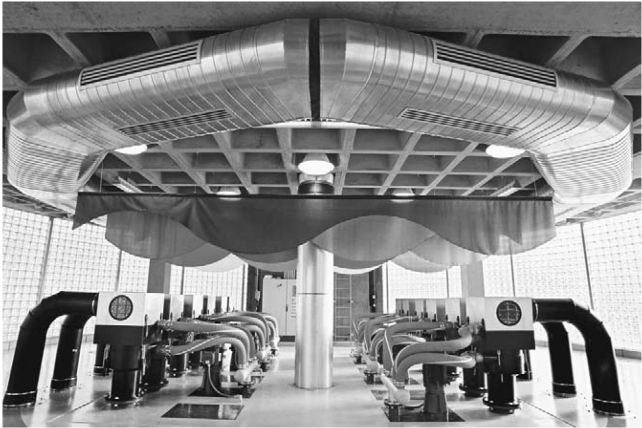
Figure 4.73 The treatment facility is housed in a 3,000-square-foot space. Image courtesy city of Wichita.
