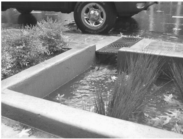
Figure 4.61 The planters are fairly simple, but they are effective at reducing stormwater runoff. Image courtesy City of Portland.
