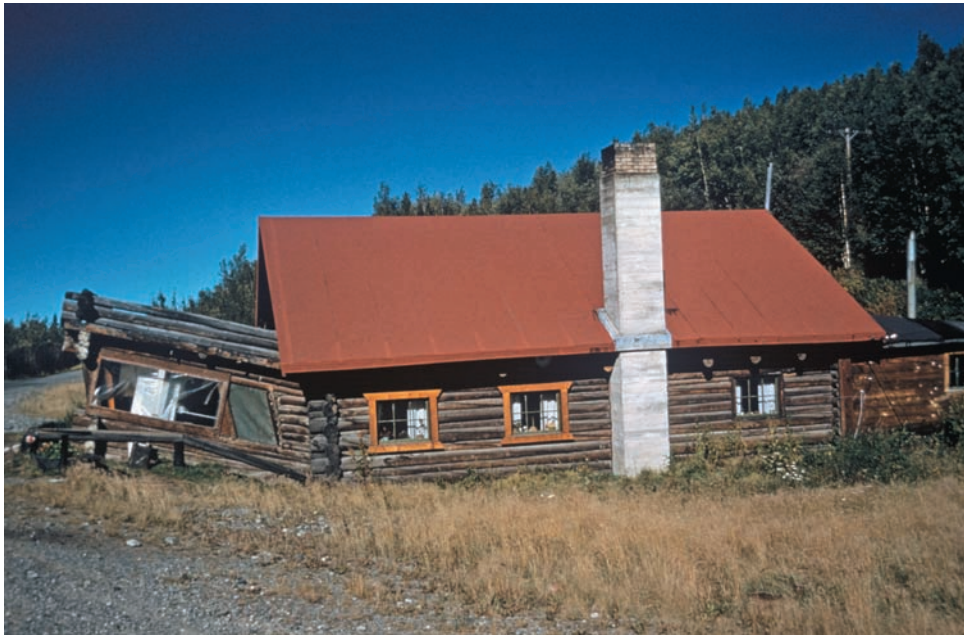
Figure 21.7 Thawing permafrost. This home is sinking as the permafrost on which it was built thaws. Thawing permafrost causes ground subsidence, erosion, and landslides. (Steve McCutcheon/Visuals Unlimited)
