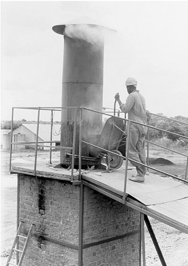
Figure 1: Loading stone/fuel through the hopper at the chimney level, lime kiln, Chegutu, Zimbabwe ©Practical Action/Kelvin Mason
