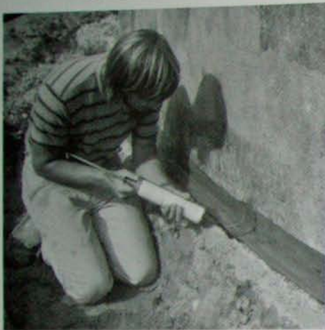
Fig. 7.1: The important waterproofing detail where the wall meets the footing is sealed with a strip of Bituthene®.
