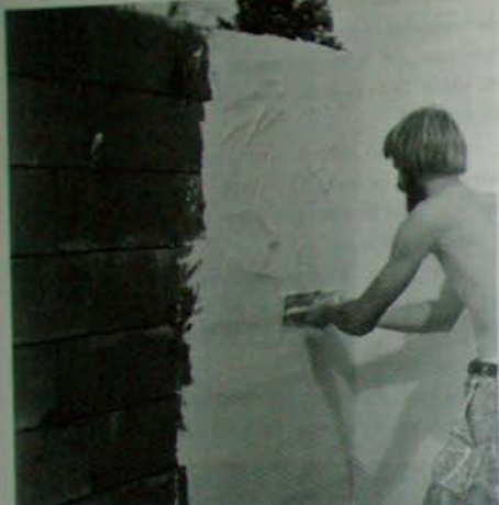
Fig. 5.8: The author presses the surface-bonding cement firmly into the dampened wall with a plasterer's trowel. pointed trowel to load up the flat trowel with SB cement. Then, beginning at the bottom of the wall, apply the mix with firm pressure on the trowel, pushing the cement upward so that a uniform covering is obtained. You can even out the plastered area and spread excess SB cement with long light strokes, always holding the trowel at about a 5-degree angle to the wall surface. Avoid over-troweling, which can cause crazing and cracking of the surface. With a little practice, you'll soon be laying a pretty consistent \frac{1}{8} -inch coating onto the wall. Until you feel confident, you can check the depth with the corner of your trowel.
