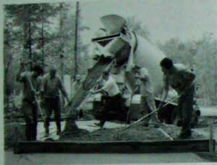
Fig. 3.7: EARTHWOOD: LAYING OUT AND DIGGING THE FOOTING TRACKS A crew of six made easy work of pouring the small four-cubic-yard monolithic floating slab at the new octagonal guesthouse at Earthwood.
