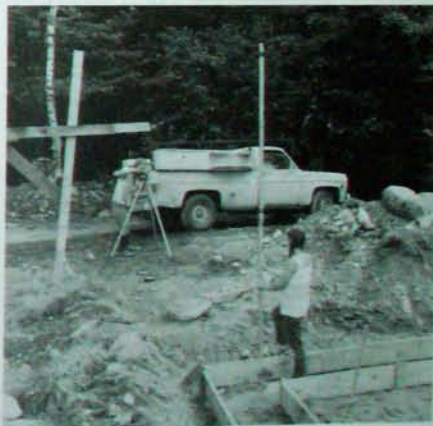
Fig. 3.11: Jaki holds a grade stake while a friend uses a contractor's level to assure that the inner and outer footing forms are all at the same grade.
