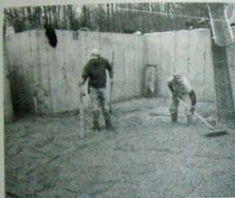
Fig. 4.14: The beam of a rotating laser level, 25 feet away, hits a grade stick. A benchmark on the grade stick shows if the concrete pad is high or low. Adding concrete or taking it away brings the pad to finished floor level.
