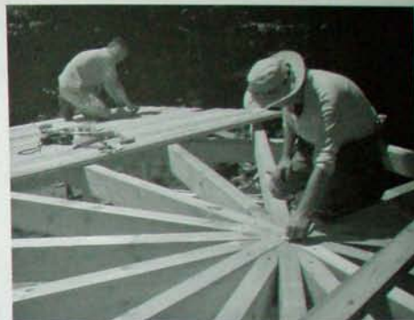
Fig. 6.18: Planking the roof at the Stoneview guesthouse was a lot like doing the Earthwood roof. Here, we snap a line on the planks, but directly over the middle of the 4 x 8" rafters. Next we cut off all the "waste" at once with a circular saw.
