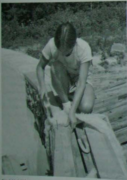
Fig. 6.16: Jaki fastens the wooden plates to the four-by-eight window lintels with 16-penny (3/4-inch) nails. To stop draft, she has installed a strip of fibreglass insulation between the plates and the lintels.
