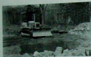
Fig. 3.5: Three or four runs of sand are built up and individually compacted, resulting in a final compacted pad of at least 18".
