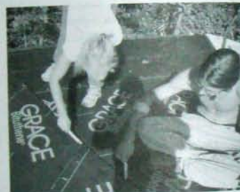
Fig. 8.3 (above): Jaki and Darin Roy leather the edge of the mastic with pointing knives, to approximate the factory edge of the Bituthene® membrane. The mastic stops the cut edge from raising up or "fish-mouthing."
