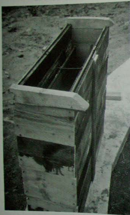
Fig. 4.16: We formed the buttresses with recycled 2 × 6" tongue-and-groove silo boards. of the sand to slow the set. And (3) Specify two trucks, maybe 45 minutes apart, so that there is no waiting for the second half of a large pour.
