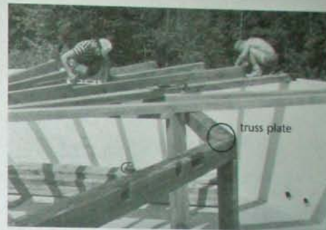
Fig. 6.15: At Earthwood, truss plates tie the girders together over the posts of the truncated octagonal frame. This internal frame cuts joist and rafter spans in half.
