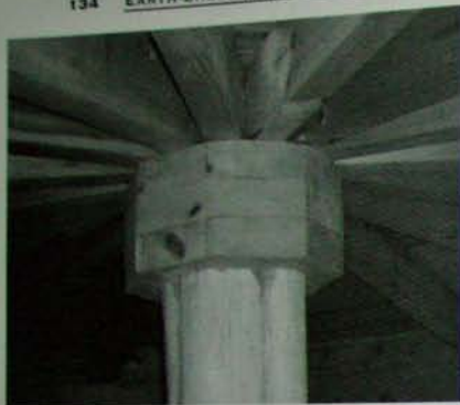
Fig. 6.14: This capital, made for the new earth-roofed Stoneview guesthouse at Earthwood, allows 16 rafters to bare comfortably on a round cedar post.
