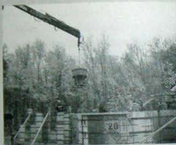
Fig. 5.1: Strong forms retain the concrete, which is delivered by chute, directly from the truck, or by hopper, controlled by the operator of the articulated boom.
