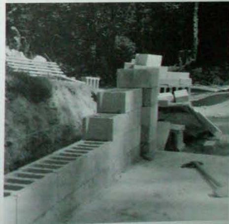
Fig. 5.7: After the first course of blocks is in place and level, build the surface-bonded wall by stacking blocks three or four courses high at each corner. Then, fill in between corners by working to a mason's line stretched from corner to corner.
