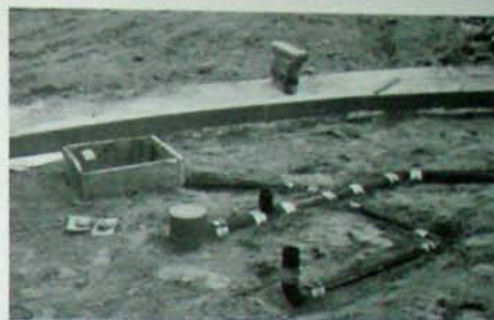
Fig. 4.9: Underfloor plumbing at Earthwood. The top of the cylindrical "red cap," mentioned in the text, is set at finished floor level, which is the same as the top of the footings.
