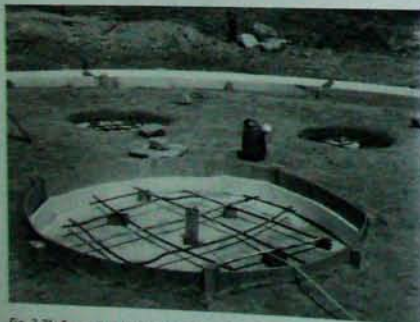
Fig. 3.21: Formed with \frac{1}{4} " plywood, the footing for the masonry stove is ready to pour.
