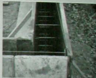
Fig. 5.2: Strong forming is critical to pouring concrete walls. Note frequent cross-ties that keep the forms from spreading.
