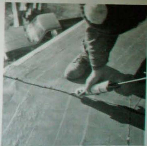
Fig. 7.9: Exposed cut edges must be sealed with a compatible caulking. After applying a bead of caulk, use a butter knife to create an edge that looks something like the factory edge. Tip: bend the last inch of a non-serrated butter knife just a little bit to make an excellent tool for this purpose.
