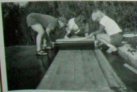
Fig. 7.6: After the sheet has been rolled back up with its backing paper on, the team again unrolls it on line, pulling the paper away at the same time. The author, on hands and knees, presses the sticky surface of the membrane onto the wooden deck.
