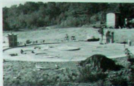
Fig. 4.5: Extruded polystyrene insulation and wire mesh are installed. The two buttresses are formed. We're ready to pour!
