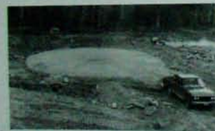
Fig. 3.6: A view of the finished sand pad at Earthwood. The pad extension near the truck is for the greenhouse.
