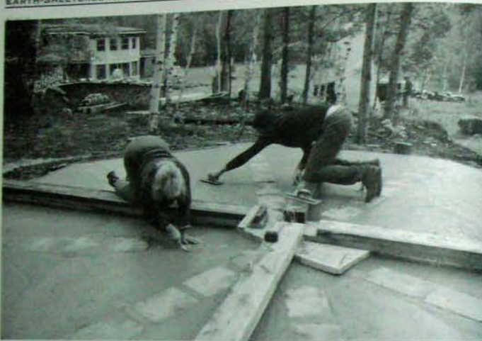
Fig. 10.4: Jaki points around slates set into the fresh concrete at Stoneview, while intern Nick Brown hand-trowels the triangular spaces between the eight slate "spokes."
