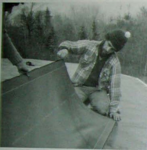
Fig. 7.8: Later, when the adjacent sheets of the same course are installed, they too should extend onto the next facet by three inches, giving a six-inch lap where two facets meet. Normally, a 3-inch lap is sufficient with Bituthene ® 3000 and 4000 membranes, but you want extra protection where facets come together, pressing hard onto three inches of solid wood on each side of the crack.
