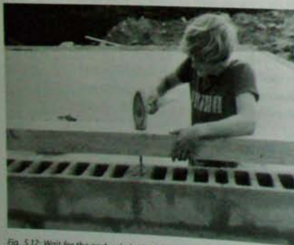
Fig. 5.12: Wait for the anchor bolts to set in the concrete plugs in the block cores. Then, locate the holes by laying the plate on the anchor bolts and whacking once sharply with a heavy hammer.
