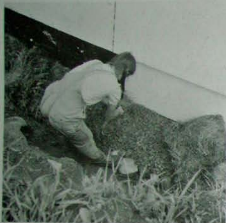
Fig. 7.15: Jaki spreads hay or straw on the crushed stone surrounding the drainage tubing.
