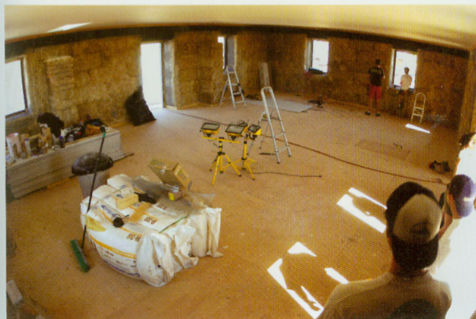
Install ceiling drywall before starting stucco work to help compress the bale walls.
