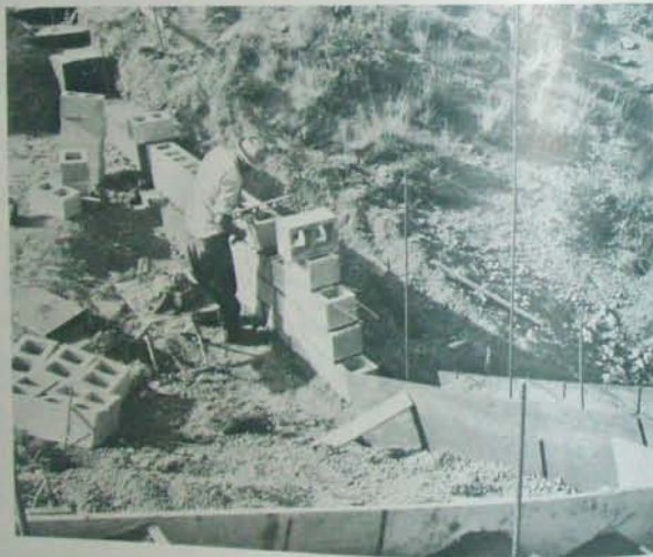
Fig. 6.3 Block stem foundations. Block, the width of adobe wall which will go above, is placed on footing and filled with concrete, making a solid stem. Note simple forms and bulkheads which provide steps in this footing for an uneven site.
