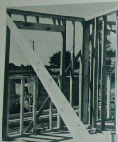
Fig. 7.19 Frame walls. Note diagonal bracing to keep walls square. Door header, cripples, trimmers, and additional blocking provide nailing surfaces at corners. Top plate is doubled to carry framing for roof above.
