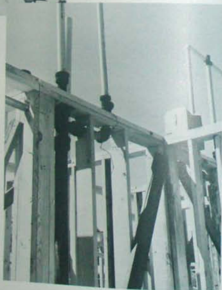
Fig. 7.20 Frame walls. Plumbing pipes are cut in notches cut in the framing. Resulting weak spots are bridged with FHA straps, which replace the original strength. If pipes are placed first, the frame wall may be built around them.
