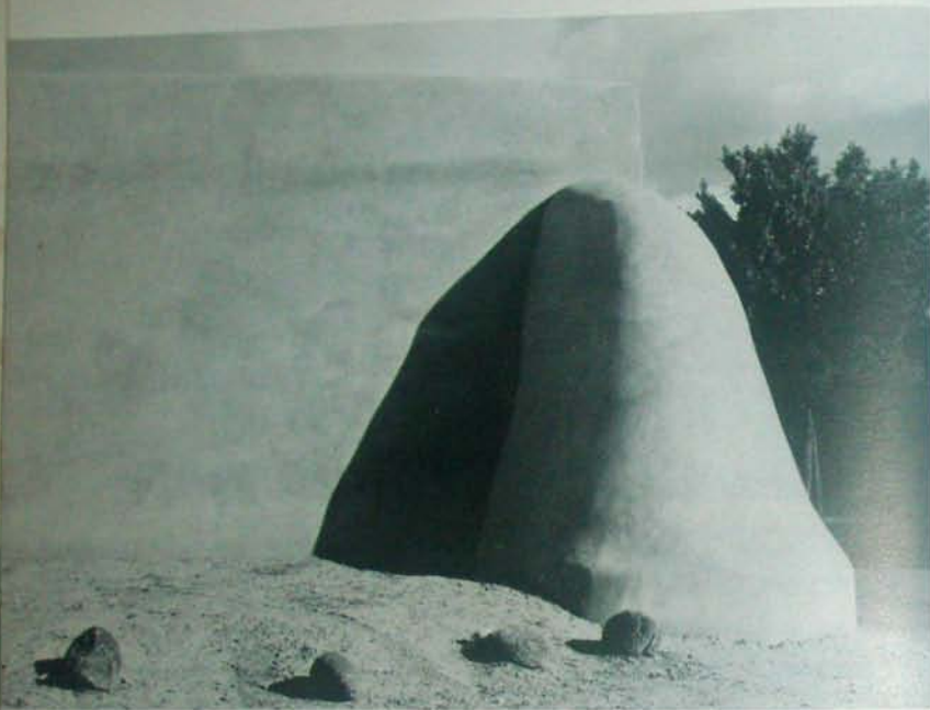
Fig. 7.9 - Ranchos de Taos Church, Ranchos de Taos, New Mexico. Masses of heavy masonry help support a corner which has started to tip, from either a lack of a bond beam or weakened foundations.
