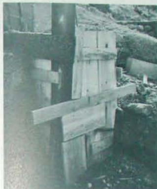
Fig. 6.4 Concrete forms. This form broke when it was filled with heavy wet concrete. The poor example above was cobbled together to contain it before it began to heave.
