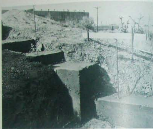
Fig. 6.2 Concrete footings. In most instances where the building site is flat, footings are contained in a trench. Where an uneven site is used, it may be necessary to step the foundations, using forms where needed, at levels which will accommodate the materials going on top of the foundation. Note vertical reinforcing rods imbedded in the footing.
