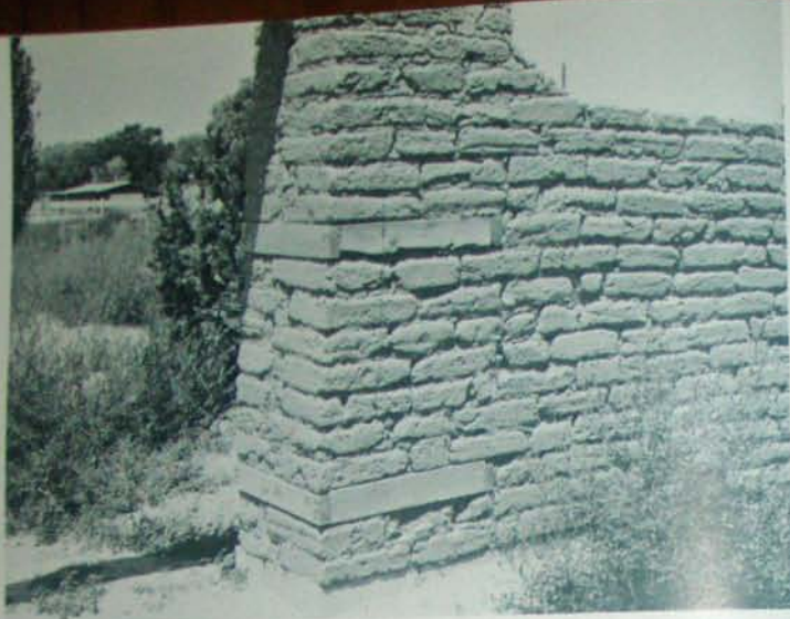
Fig. 7.7 Adobe wall with "gringo" blocks, block stem. Wooden "gringo" blocks have been set in place of adobes to provide anchorage for doors, windows, or as in this case, a gate. This wall has been exposed to the weather for approximately five years with little damage. Note concrete blocks extending above ground level, preventing ground water from damaging bottom of wall.
