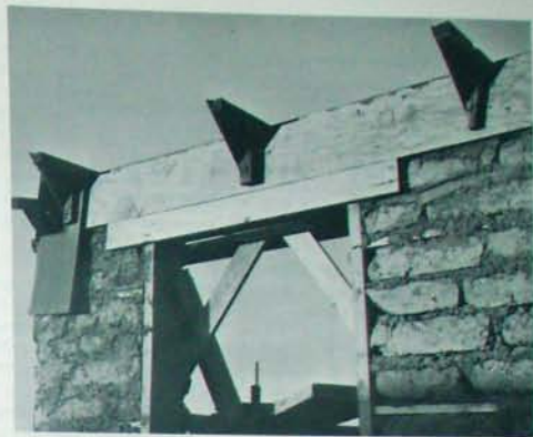
Fig. 7.11 - Bond beam form. Form may be held in place with simple metal brackets. A patching piece is used at windows and doors to cover the thicker lintel. Note 1 x 4 nailer strips laid up with the adobe wall, in place of "gringo" blocks.
