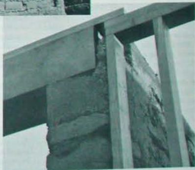
Fig. 7.13 - Grand Junction, Concrete bond beam, heavy timber lintel, and frame wall all come together at one corner. Note support for timber lintel (concrete pad atop adobe wall).
