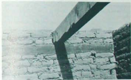
Fig. 7.12 - Bond beam. Form has been stripped off, vigas placed, and adobes continued above bond beam.
