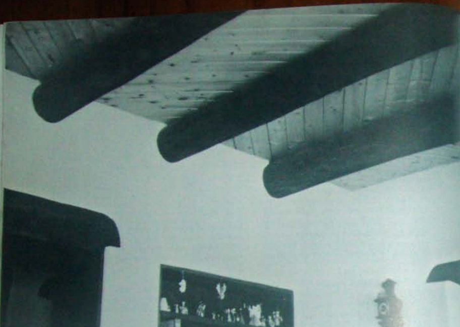
Fig. 9.1 Residence, Corrales, New Mexico. Traditional round vigas contrast with exposed tongue-and-groove decking. Note herringbone effect which can also be achieved through the use of latillas or sedros.
