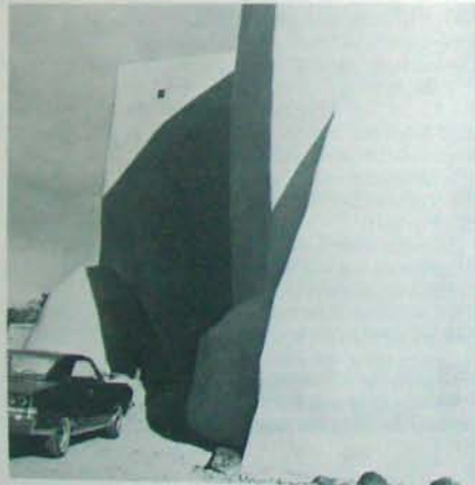
Fig. 7.10 - Ranchos de Taos Church, Ranchos de Taos, New Mexico. High walls may also need some support.
