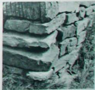
Fig. 6.5 Rock foundations. Have been used traditionally with great success before the invention of ready-mix concrete plants. If using this method, it is best to make sure the rocks fit well without mud mortar, which may melt under severe rains.
