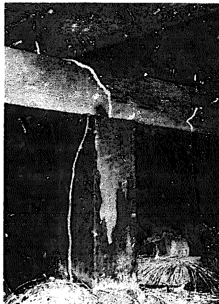
Subterranean Termite tunnels running up a house stump
