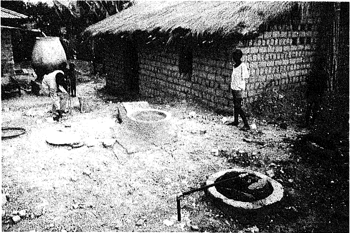
Photo 10: Fixed-dome biogas plant. Inlet at left, entry hatch/gas outlet at center, displacement pit and slurry store at right (Source: OEKOTOP)
