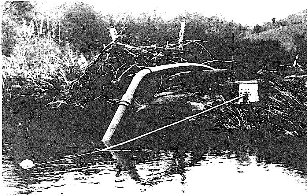
Photo 5 — Siphon intake and water meter at the reservoir
