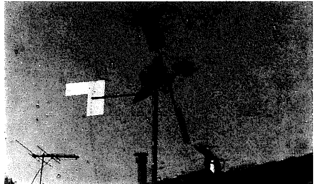
Owner-built wind generator
