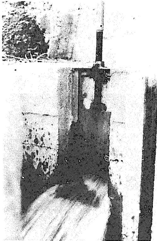
Figure 7.20: Gate valve in open conduit
