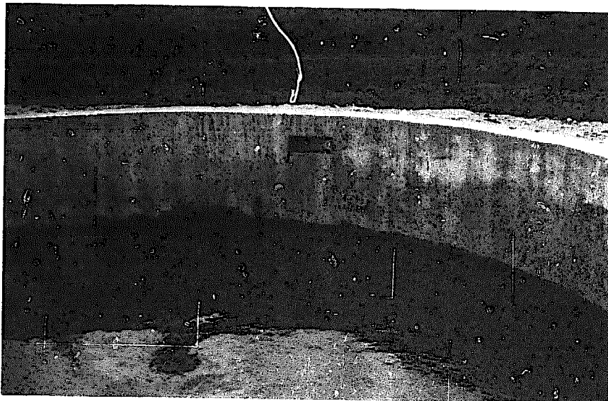
Fig. 12 Water inlet installed in a diagonal position on the wall of a spawning tank to circulate water, Pai-tan Lake Fish Cultivation Station
