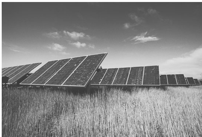
Figure 8-8 Vallejo photovoltaic installation. (Courtesy: BP Solar.)
