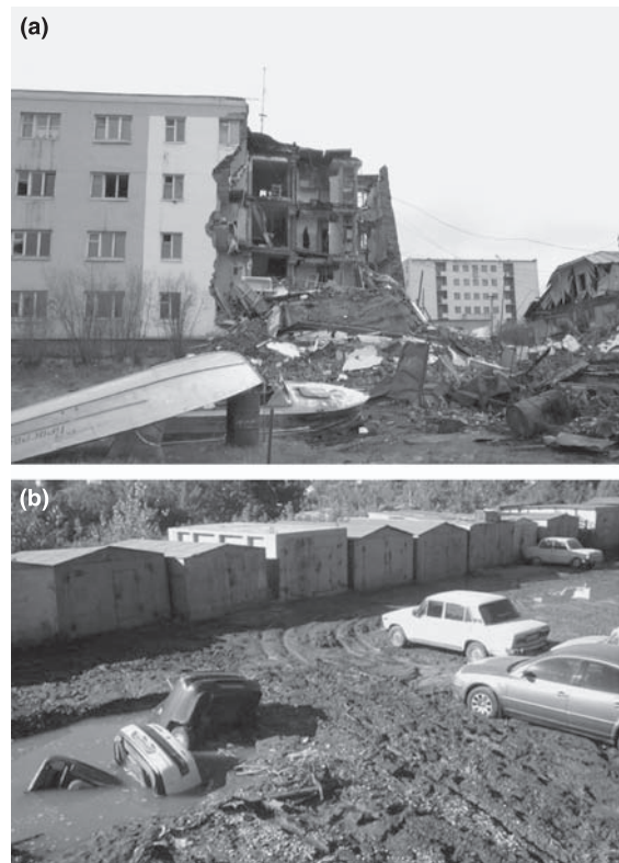
FIGURE 13.7. Damages provoked by permafrost thaw in Russian cities. (a) Collapse of a section of a residential building in Cherskiy, East Siberia, due to thawing of permafrost (photo by V. E. Romanovsky). (b) Extensive thermokarst development in a car park lot in Yakutsk (photo by N. Shiklomanov).
