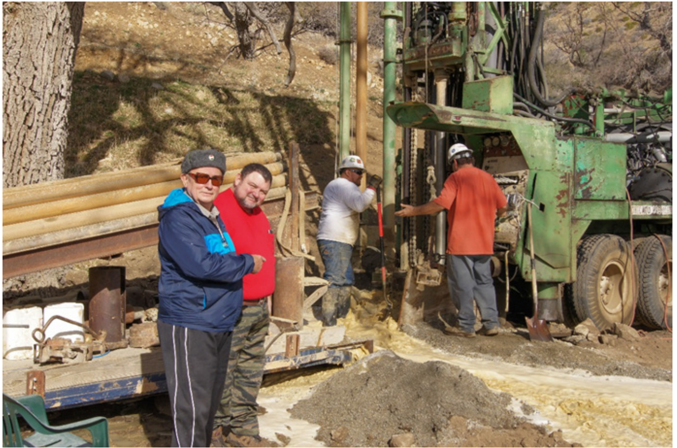
Pal and Ben with the drillers. Water and debris encountered at 50 feet at final phases of drilling.
