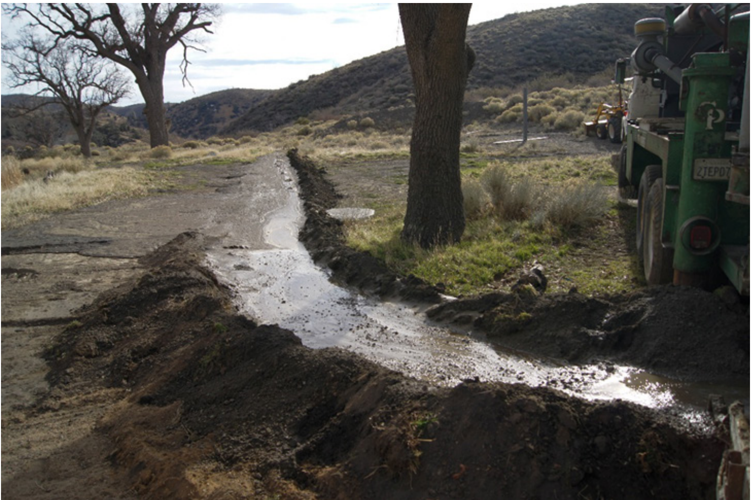
Water flow discharged in trench. Estimated output of water is 800 gallons plus per minute. Unable to drill borehole beyond 65 feet due to large volume of discharged water and debris/cuttings.
