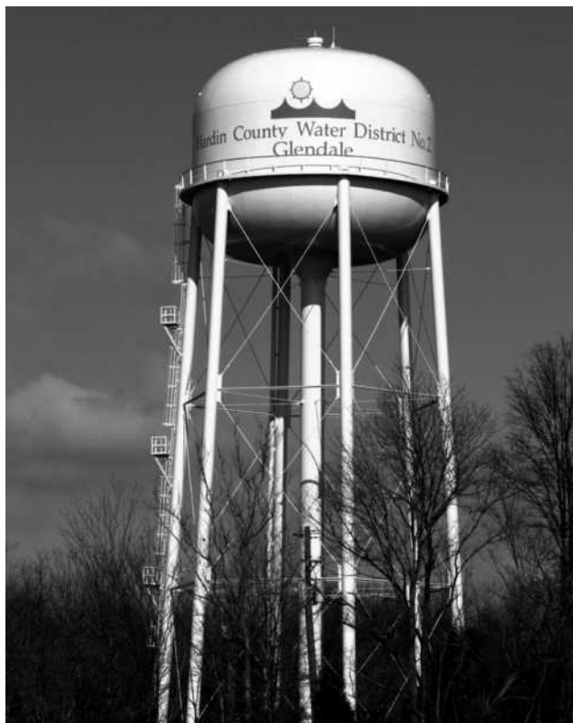
Figure 2. Traditional multicolumn elevated storage tank (Source: Caldwell Tank, Inc.)
