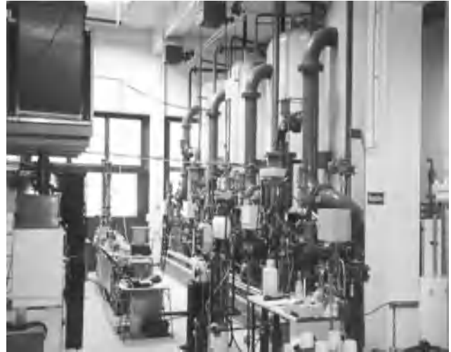
Figure 2. Pilot plant unit, which was used for the biological oxidation and removal of iron and manganese (Umweltbundesamt, Institute for Hygiene of Water, Soil and Air, Berlin, Germany).
