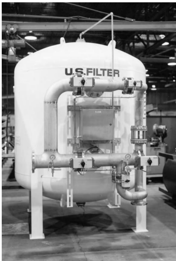
Figure 3. Pressure filter (Source: U.S. Filter).
