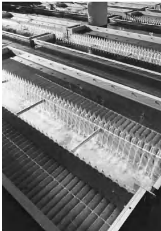
Figure 4. Installed plate settlers (Source: U.S. Filter).
