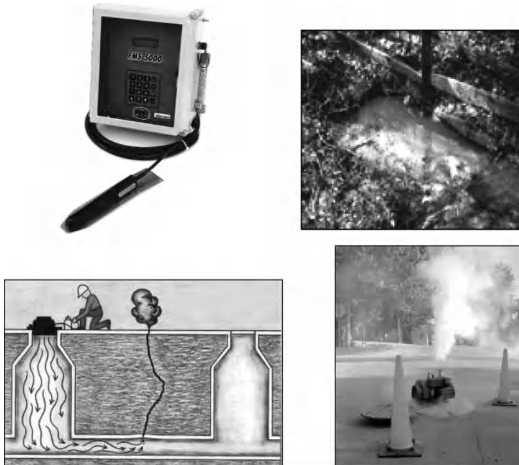
Figure 4. Flow monitoring device, dye testing, and smoke testing in sewers (clockwise from top left).
