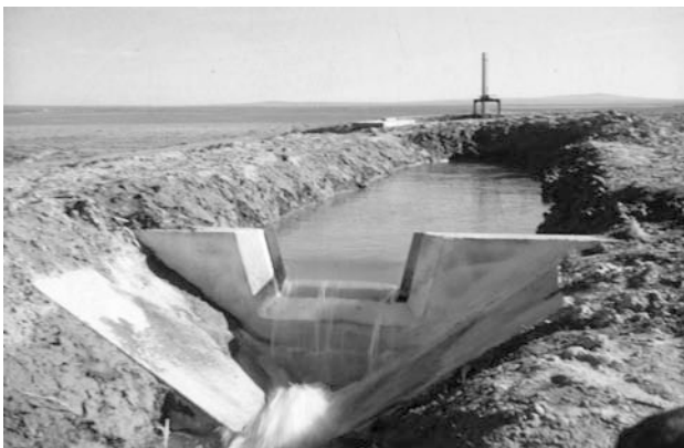
Fig. 3 Trapezoidal weir installed in an earthen channel.
