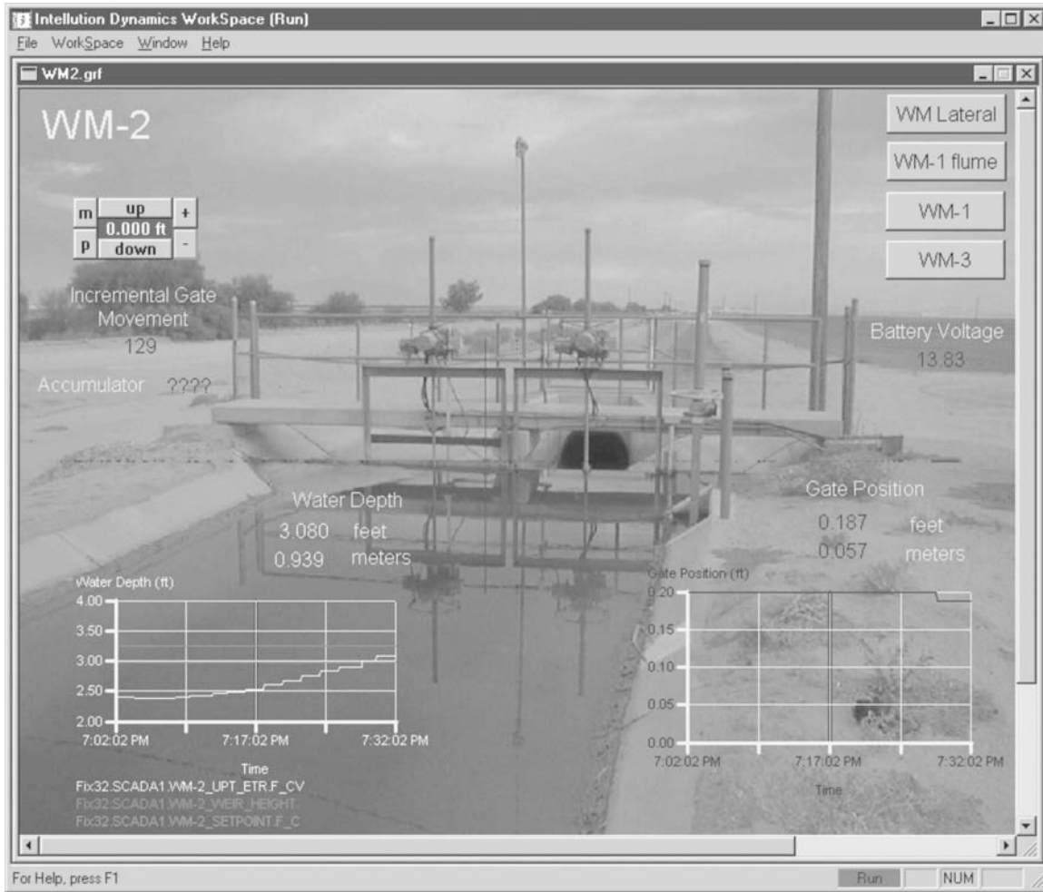
Fig. 1 Check structure with motorized check gates and a manual outlet gate shown as part of SCADA automatic control screen.
