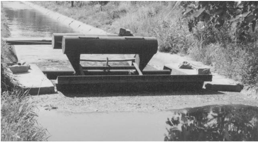
Fig. 3 Amil gate for constant upstream level control.
