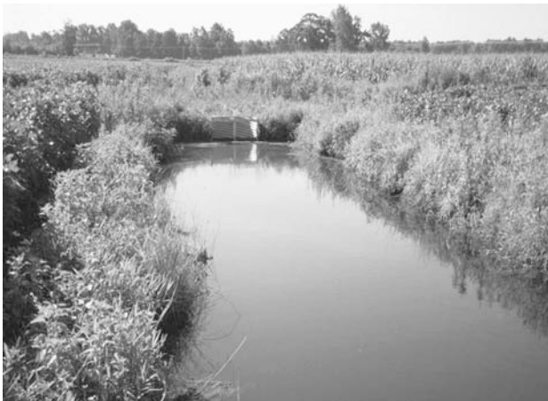
Fig. 2 Flashboard riser type water control structure used to manage the outlet water level in an open ditch system.
