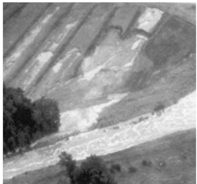
Fig. 8 Erosion damage of an auxiliary spillway after experiencing a flow.
