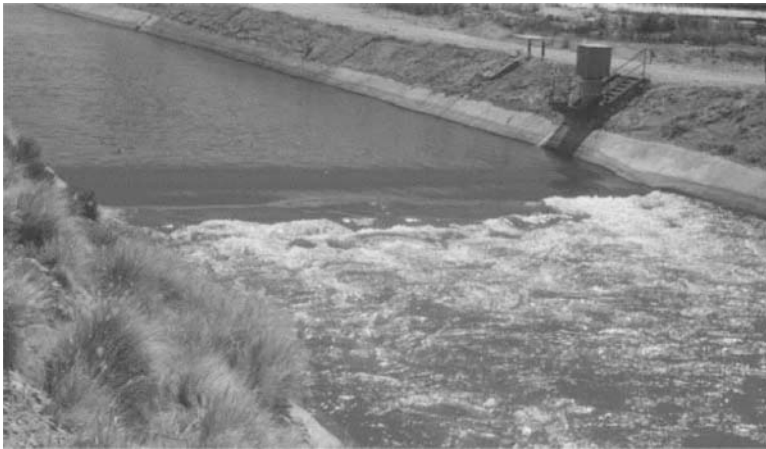
Fig. 1 Flume in large canal. Note stilling well and the region of wavy water surface. Sill crest is located about midway between these two features. Canal flow depth is about 2.4 m (8 ft) and sill crest is about 1.4 m (4.5 ft) high.
