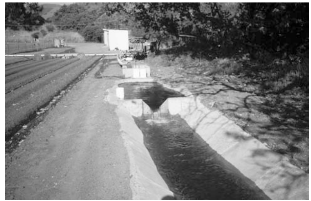
Fig. 4 Flume installed in a small concrete channel.
