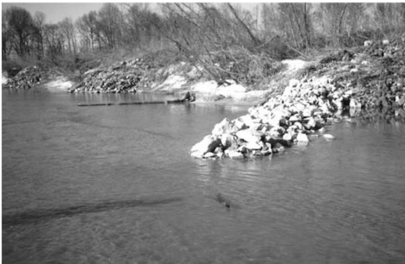
Fig. 3 Stone spur, a form of indirect protection, used to deflect erosive flows away from bank. Spur was made from quarried riprap.
