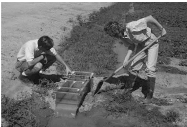
Fig. 2 Adjustable flume being installed while channel continues to flow. Capacity 56 L/sec (2 cfs).
