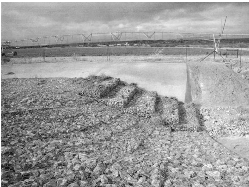
Fig. 1 Stair stepped gabions, wire mesh, and concrete reinforced bank controlling erosion on the edge of an irrigated field in southern Arizona.
