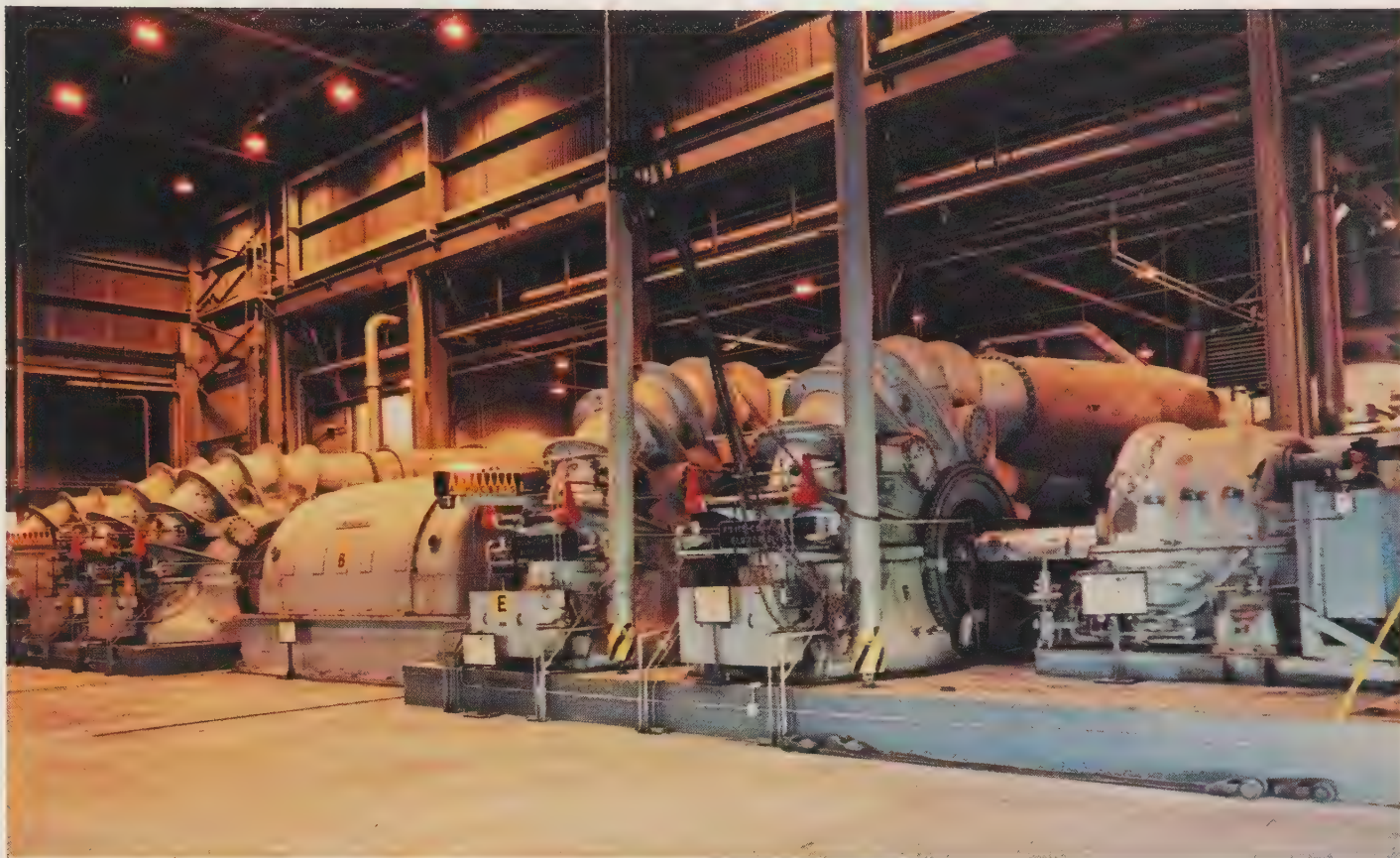
Under the Unitary Plan, Langley built a supersonic tunnel with two test sections that spanned Mach numbers 1.5 through 4.6. Shown here is the battery of six compressors needed to supply compression ratios between 1.3 and 16. The corresponding family of electric-drive motors was rated at 100 000 horsepower.
