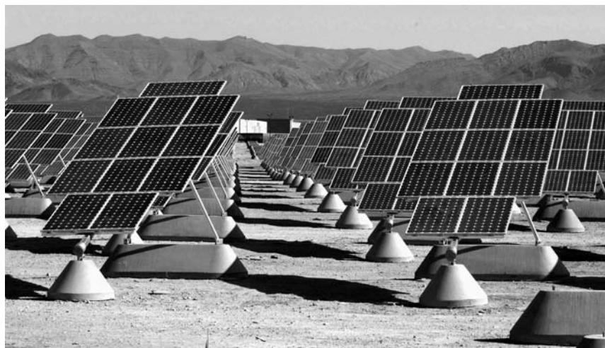
The solar field at Nellis Air Base in Nevada has more than 72,000 panels and supplies the base with more than 30 million kilowatt-hours of power.
