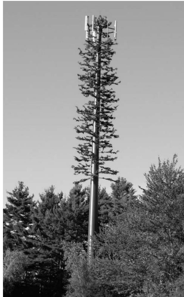
A cell phone tower disguised as an evergreen tree. Cell signals are sent through towers via radio signals.
