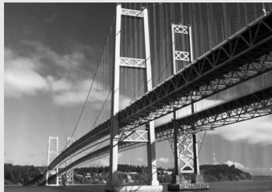
The Tacoma Narrows Bridge
