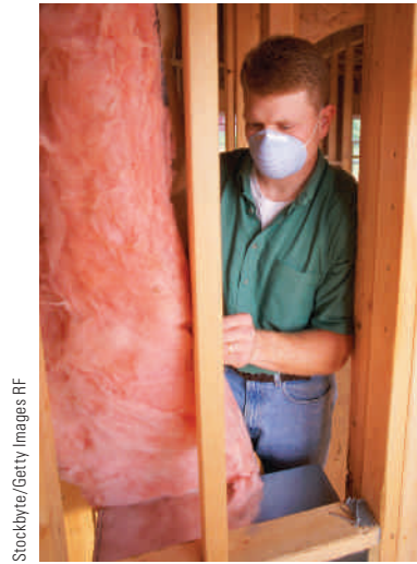
A worker installing fiberglass insulation in a home. The mask protects the worker against the inhalation of microscopic fibers, which could be hazardous to his health.
