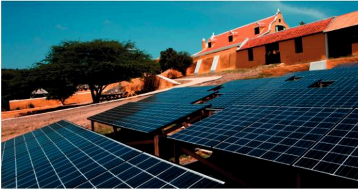
▲ Figure 7.11.2 Photovoltaic cells in a natural reserve park in Curacao
