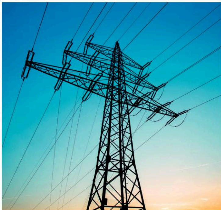
▲ Figure 18.6.3 Power lines
