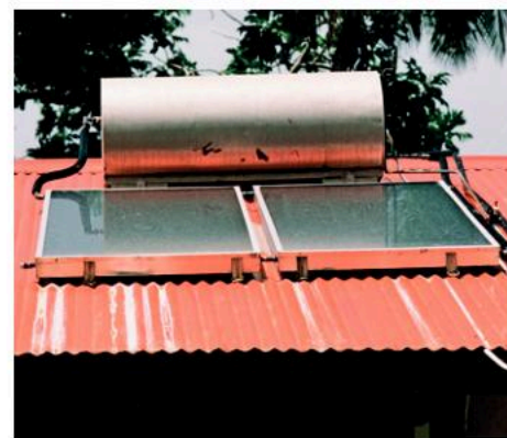
▲ Figure 8.4.8 Solar water heater on the roof of a building in Barbados. It comprises two rectangular plate collectors and, above those, a cylindrical water storage tank. Inside each collector are a series of small tubes that pass over a black absorber plate. The plates absorb sunlight and warm the water passing through the tubes. Warmed water rises to the storage tanks by convection as it is heated. Colder water sinks down into the collector. This system, known as a thermosiphon solar water heater, is cheap to install and maintain, and produces no waste products.
