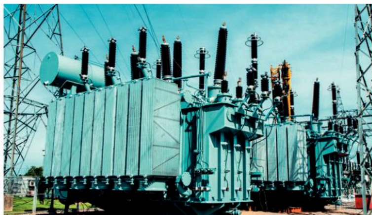
► Figure 14.10.2 Transformers at an electricity substation
