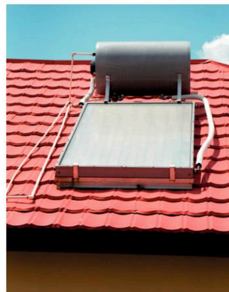
▲ Figure 15.3.3 Solar water-heating panel mounted on the roof of a house in Kingston, Jamaica
