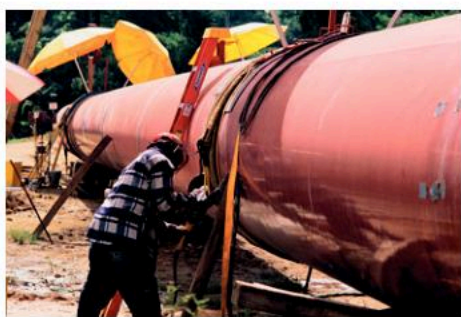
▲ Figure 20.5.4 The technician is checking the join in a gas pipe line for flaws or poor welding. Photographic film is mounted on the inside of the pipe with a radiation source on the outside. The photograph was taken in Trinidad and you can see parasols used to provide shade for the workers.
