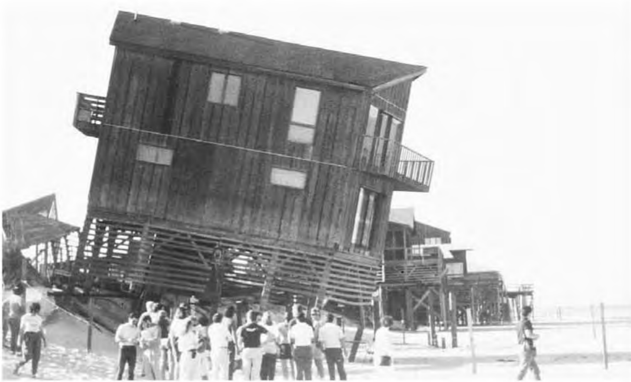
Beach erosion can adversely affect near-shore structures such as this one on the Outer Banks of North Carolina; this erosion was caused not by a hurricane, but by a Noreaster—a low-pressure system that can form over the eastern U.S., where moist Atlantic air feeds the storm to create high levels of precipitation and strong winds. NOAA/Richard B. Mieremet, Senior Advisor, NOAA OSDIA
