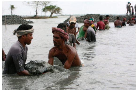
Figure 13.9 Bangladeshi villagers rebuild an embankment at Protap Nagar in Shatkhira, about 176 km southwest of Dhaka, Bangladesh, on Sunday, 31 May 2009. Hundreds of thousands of people in eastern India and Bangladesh were flooded out of their homes by Cyclone Aila, with many crowded into government shelters. Photograph from Press Association/Pavel Rahman.
