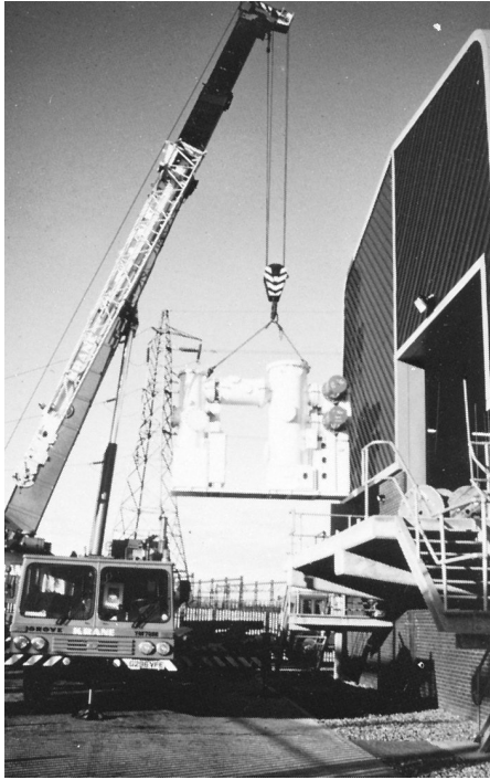
FIGURE 2.61 (Photo courtesy of the Institution of Electrical Engineers.)
