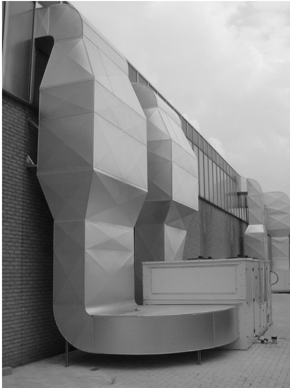
Figure 25.3 Air-handling units providing air conditioning for production plant, total installed capacity 145 kW (Johnson Controls)
