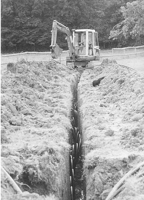
Figure 27.2 Trench for ground source heat pump showing pipe through which glycol solution will be circulated to collect heat (Kensa)
