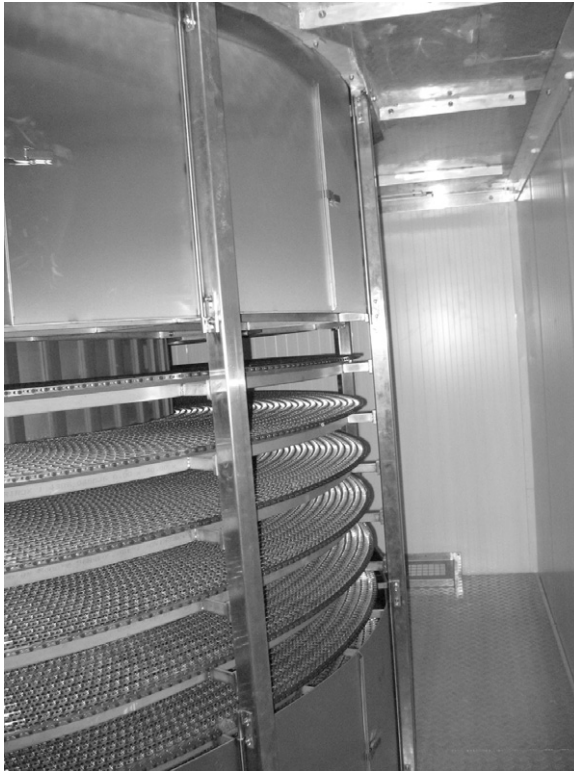
Figure 14.2 View of spiral freezer (Star Refrigeration)
