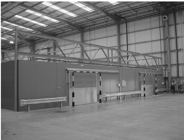
Figure 17.8 Refrigerated compartment within a warehouse for a range of frozen and chilled products (Star Refrigeration)
