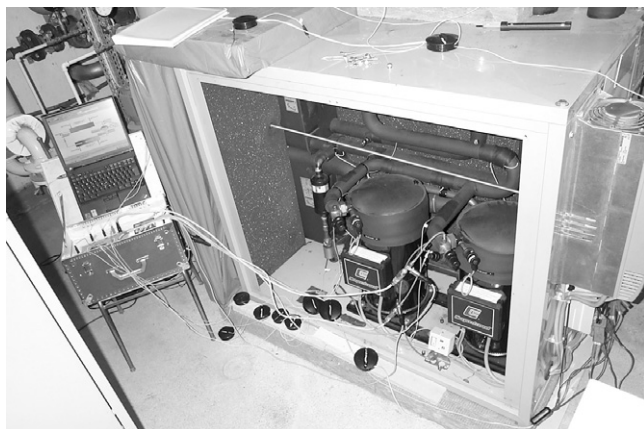
Figure 29.1 Field performance analyser connected to heat pump unit (Climacheck)
