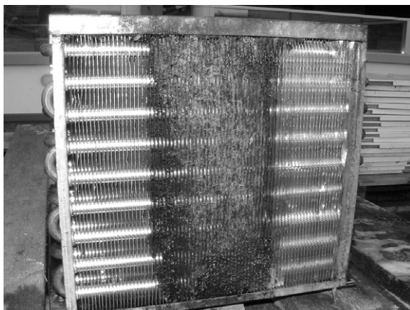
Figure 29.3 A typical condenser before and after cleaning (Advanced Engineering)
