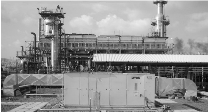
Figure 19.1 Refinery control room cooling, 390 kW total cooling capacity (Johnson Controls)
