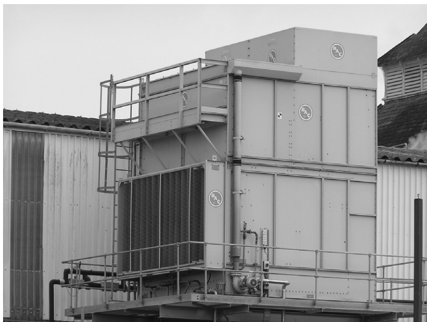
Figure 6.8 Evaporative condenser installation (Baltimore Aircoil)
