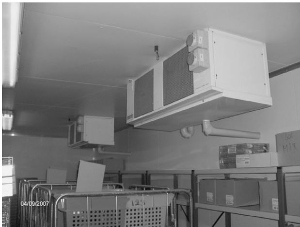
Figure 15.8 Ceiling-mounted coolers (Michael Boast)
