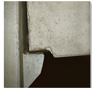
This concrete girder rests on the ledge that is assumed to act as a smooth contacting surface. (6)
