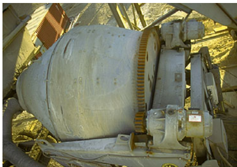
The work of the torque or moment developed by the driving gears on the motors is transformed into kinetic energy of rotation of the drum.
