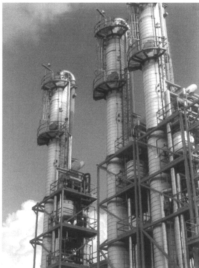
Figure 6-3. Vertical vessel. Courtesy of Nisseki Chemical Texas, Inc., Bayport, Texas.
