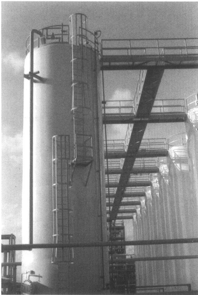
Figure 6-5. Ladder, cage, and platforms. Courtesy of Nisseki Chemical Texas, Inc., Bayport, Texas.
