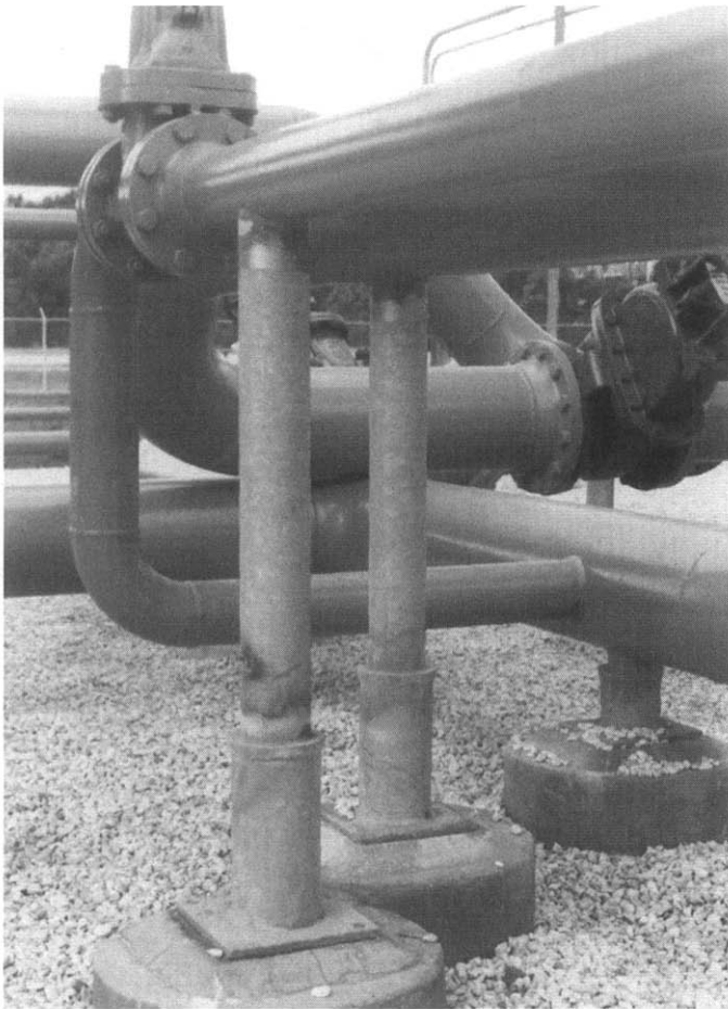
Figure 11-12. Field support. Courtesy Nisseki Chemical Texas, Inc., Bayport, Texas.
