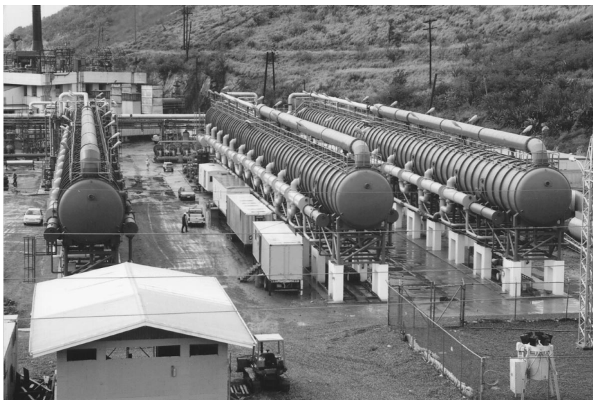
FIGURE 20.6.3 Two HTME desalination units, each producing 5000 m 3 /day, in St. Croix, U.S. Virgin Islands. (Courtesy of I.D.E. Technologies Ltd.)
