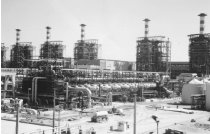
FIGURE 4.1.2 One of the six units of the 346,000 m 3 /day MSF desalination plant Al Taweelah B in Abu Dhabi, United Arab Emirates. (Courtesy of Italmimpianti S. p. A.) It is a dual-purpose plant, composed of six identical power and desalination units. Five of the six boilers are seen in the background. The desalination units were in 1996 the largest in the world. They have 17 recovery and 3 reject stages and a performance ratio (PR) of 8.1. The plant also produces 732 MWe of power.
