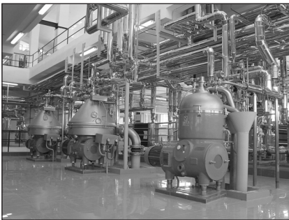
FIGURE 8–41 A piping network in an industrial facility.
